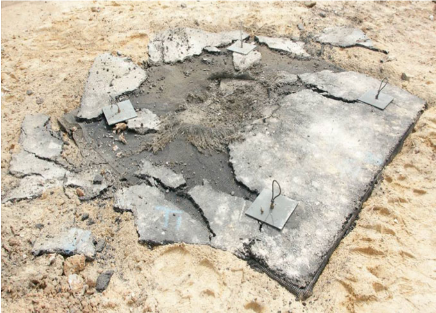
Fig. 5.41 Damage of proposed multi-layer pavement after blast
