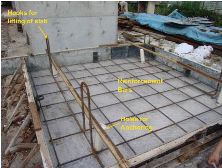
Fig. 3.4 Minimal reinforcement at bottom of slab
