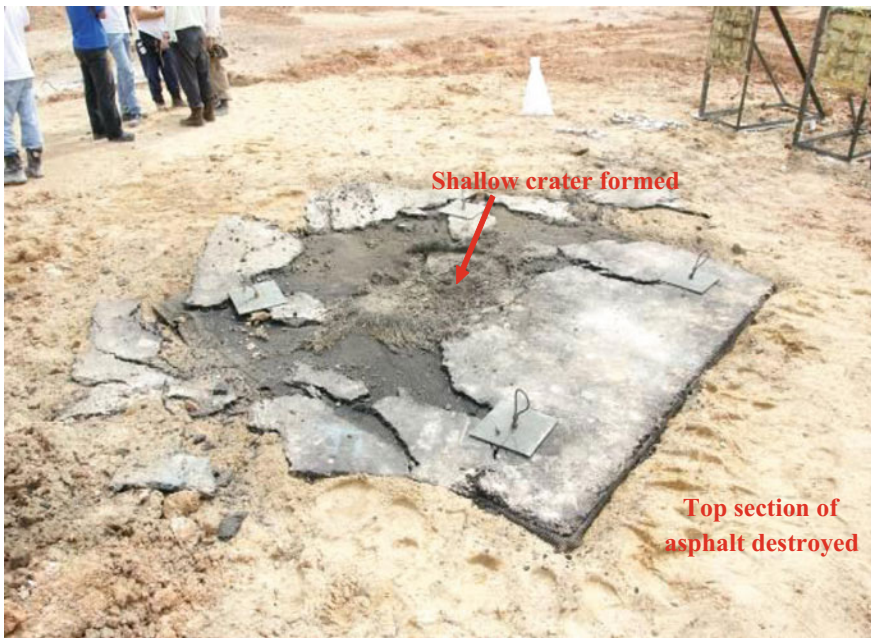
Fig. 3.35 Damaged pattern of the Slab 2 after blast
