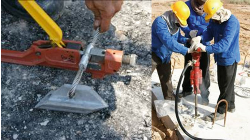
Fig. 3.9 Attachment of steel cable to anchor and driving in of the anchor using an air compressor
